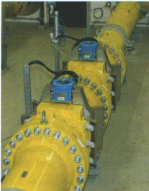
Figure 5: USZ 08 of RMG by Honeywell installed in a tandem arrangement in a gas metering station for an underground storage facility in Germany
